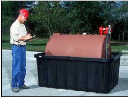
Temporary secondary containment without cover
